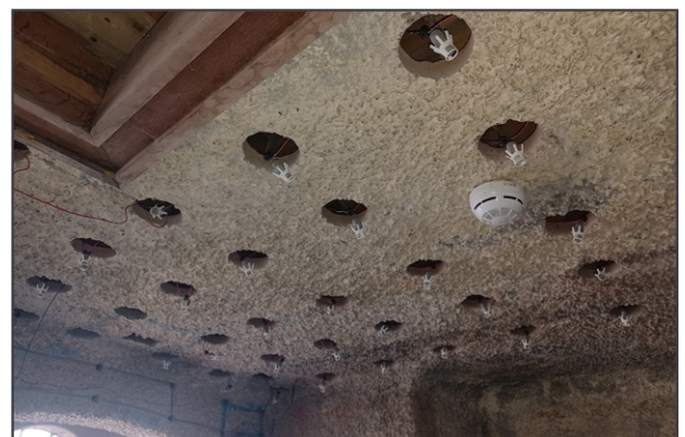
Angled anodes to ceiling
