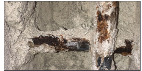
Example of corrosion in RAAC
