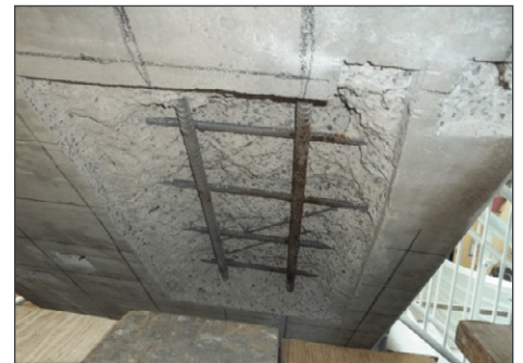
Corrosion under staircase
