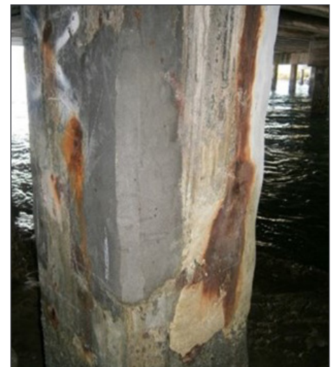
The structural problem identified
