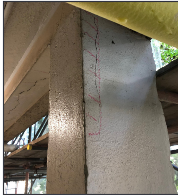
Cracking and delamination
