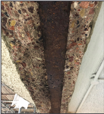
Corrosion of beam flange
