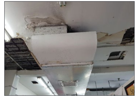
Spalling to soffit below car park.
