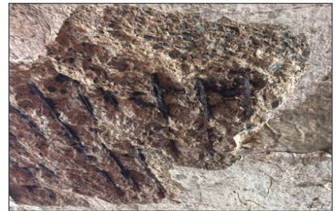
Spalling found on the soffit concrete
