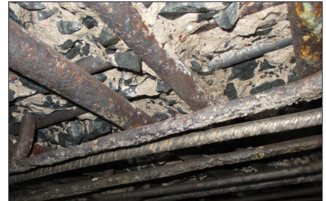
Corrosion on the structural steel reinforcement
