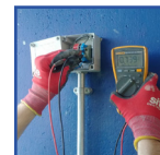
CPT Monitoring System
