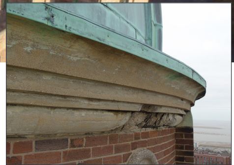
The structural problem identified
