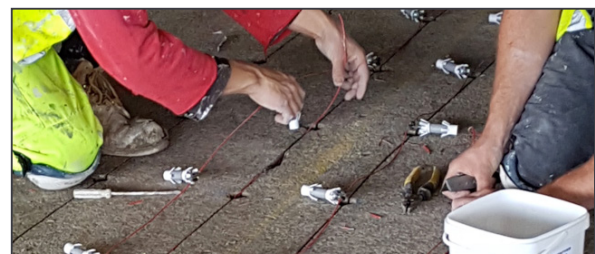
Extensive concrete damage on car park deck and DuoGuard installation.
