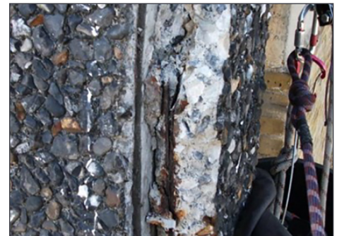
Spalling found on the pre-cast panels
