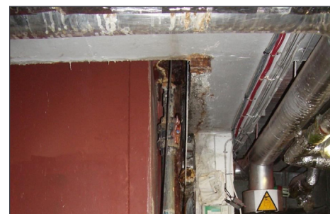
Chloride corrosion to the underside of the pool
