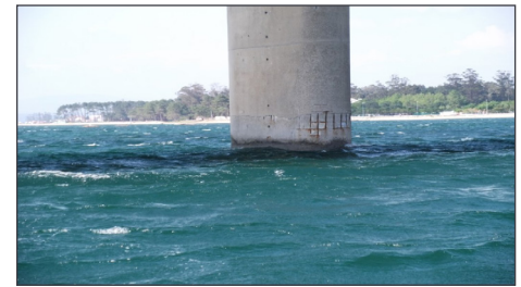
Steel corrosion in the piers
