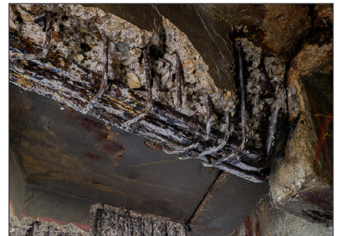
Severe deterioration, Abercorn Bridge
