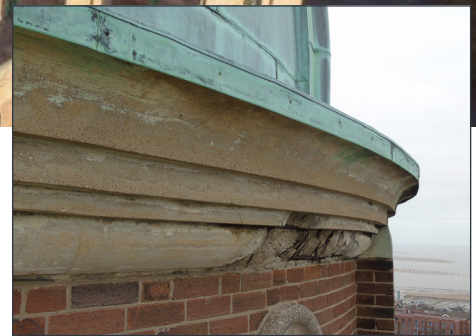
The structural problem identified
