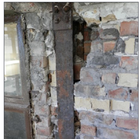
Corrosion found on the rear brickwork face of the building
