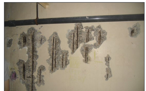
Corrosion found on the pool walls and walkway soffits
