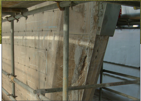
Visible spalling and loose concrete
