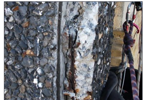
Spalling found on the pre-cast panels
