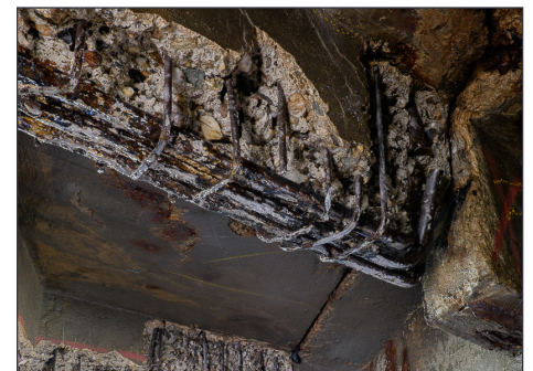
Severe deterioration, Abercorn Bridge
