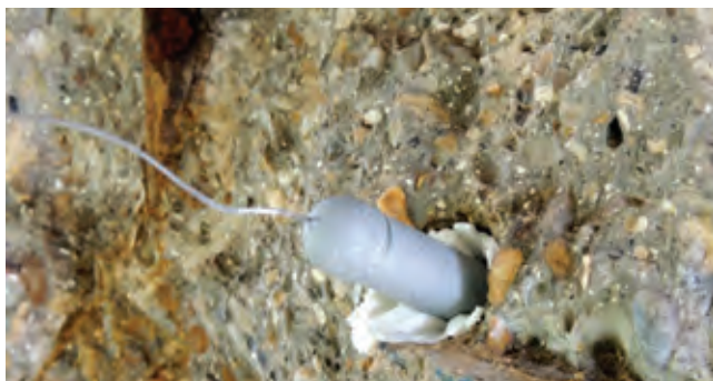
▶ PatchGuard anode being installed at the edge of the patch repair area
