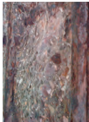
Corroding steel in concrete
