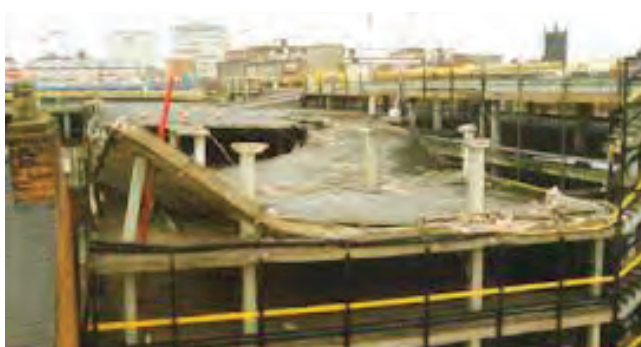
▶ Concrete deterioration caused the collapse of Pipers Row carpark
