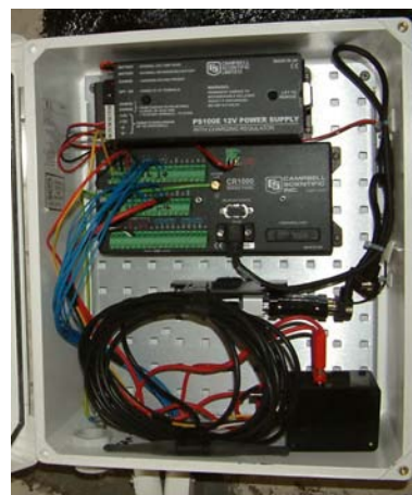
On-site Data-logging box
